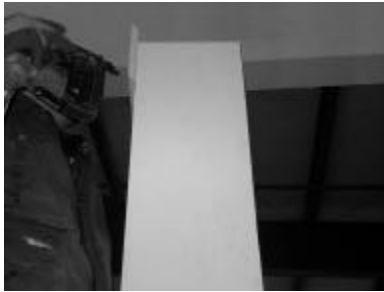
17) There are TWO methods of attaching the cap. First, apply adhesive to mitered ends of cap moulding (7¼" tall) and assemble around shaft. Screw or nail joints.
