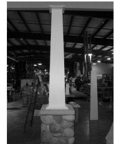
18) Clean surface of column with cleaner recommended by the paint manufacturer. Paint with 2 coats of acrylic latex paint.
