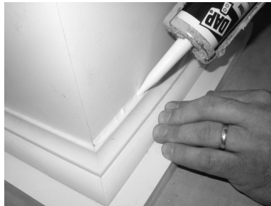
17) Caulk using latex caulking compound to fill any gaps and nail or screw holes.
