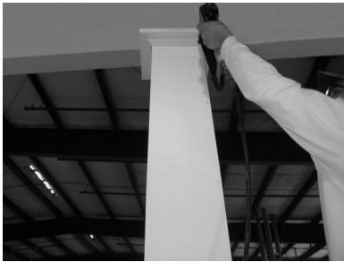
13) Apply glue to final 1/4 cap piece and biscuits and slide into place. Pin nail cap moldings to top of column.*
