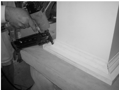
16) Center trim moldings around shaft. Apply adhesive to base trim moldings and pin-nail into base platform. (Do not attach to shaft.) There should be about a 1/16" gap around shaft.
